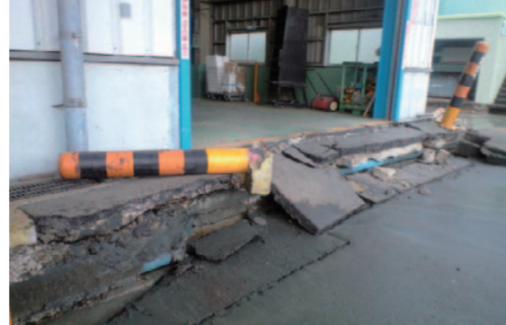
Land subsidence by liquefaction of land
