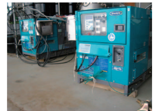
The two generators supplied by the Matsusaka Plant
